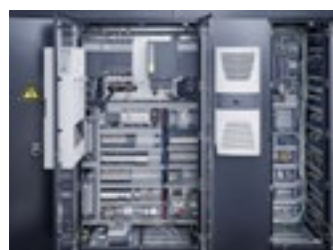
• Climatised electrical cabinet. • Automatic programable central lubrication system.
