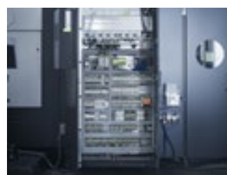
Climatized electric cabinet with easy access.
